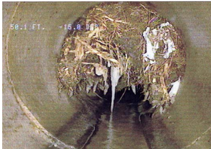
Severe Root Intrusion – Right Grease Buildup - Bottom
