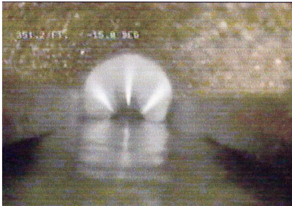
Crown Corrosion in a Concrete Pipe Hydraulic Jet Cleaner in the background
